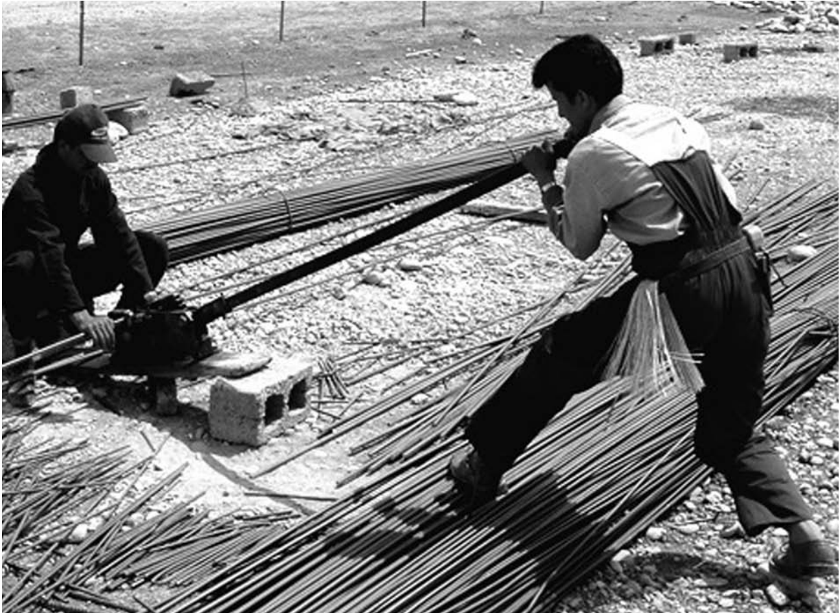
Iraqi subcontractors cut rebar for a health care clinic under construction outside of Erbil, Iraq, 20 June 2005. The clinic will handle primary health care requirements for a suburban neighborhood outside of Erbil. The U.S. Army Corps of Engineers oversees the project and works directly with Iraqi workers and contractor companies.
